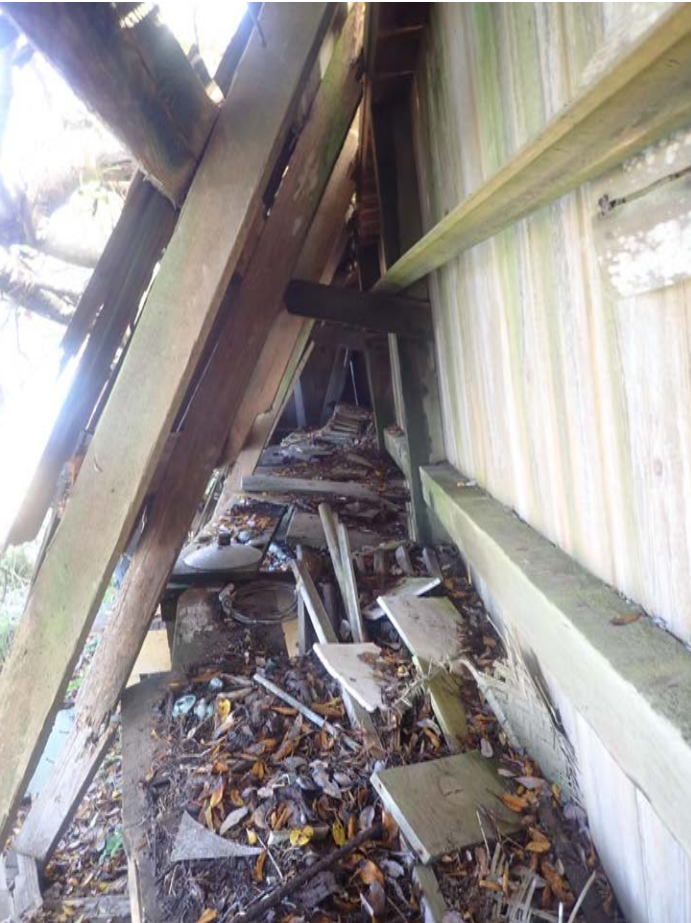
Figure 2. Another view of the collapsed coop.
