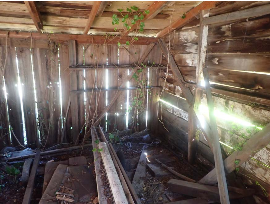
Figure 4. The interior of the carriage house was already relatively drafty.
