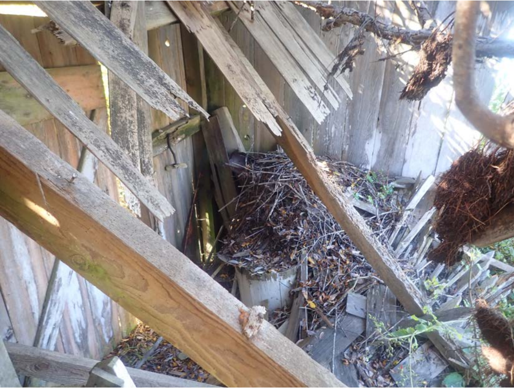
Figure 1. Old chicken coop with collapsed wall.
