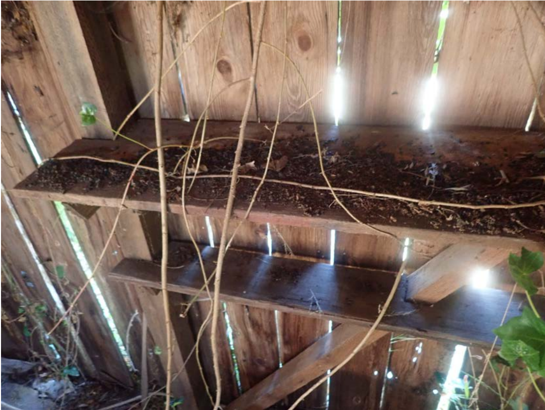
Figure 5. Woodrat droppings present in carriage house.
