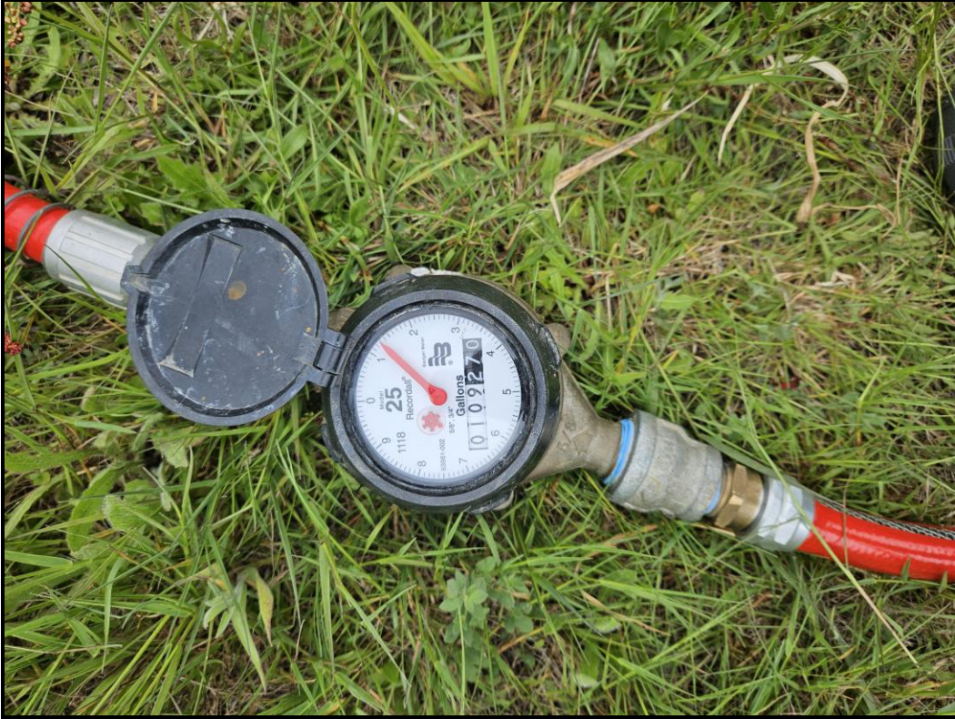
Photo 4: View of totalizing flow meter used to measure flow rate and volume.
