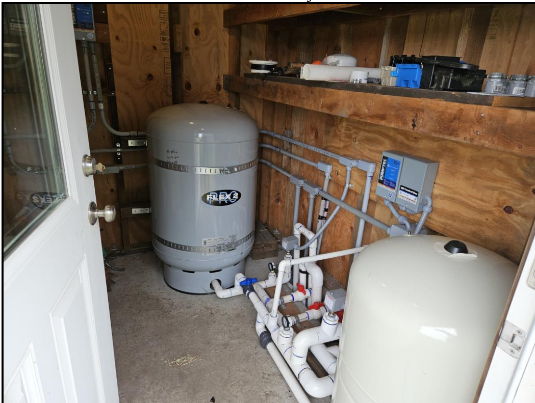
Photo 3: View inside well house located next to Site well.
