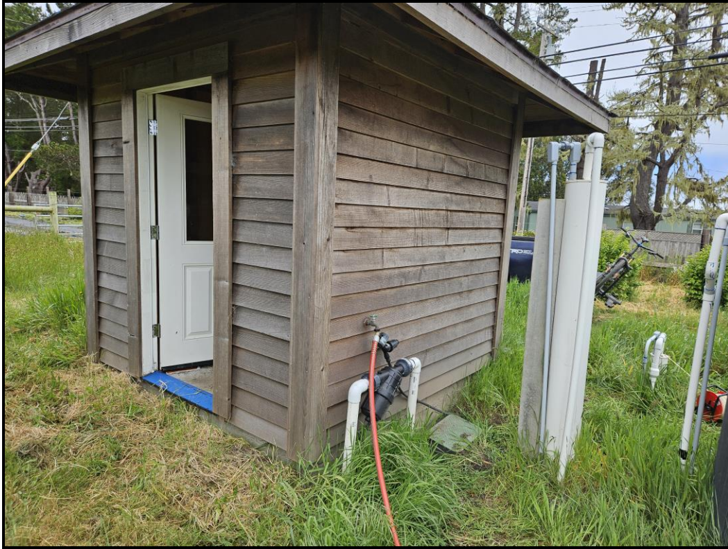
Photo 2: View of well house located adjacent to the Site well.
