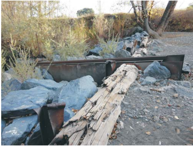
Photo B: Photograph of the two rows of wooden piers. Note the excavation of the buried gas pipeline in the upper left corner of the picture.
