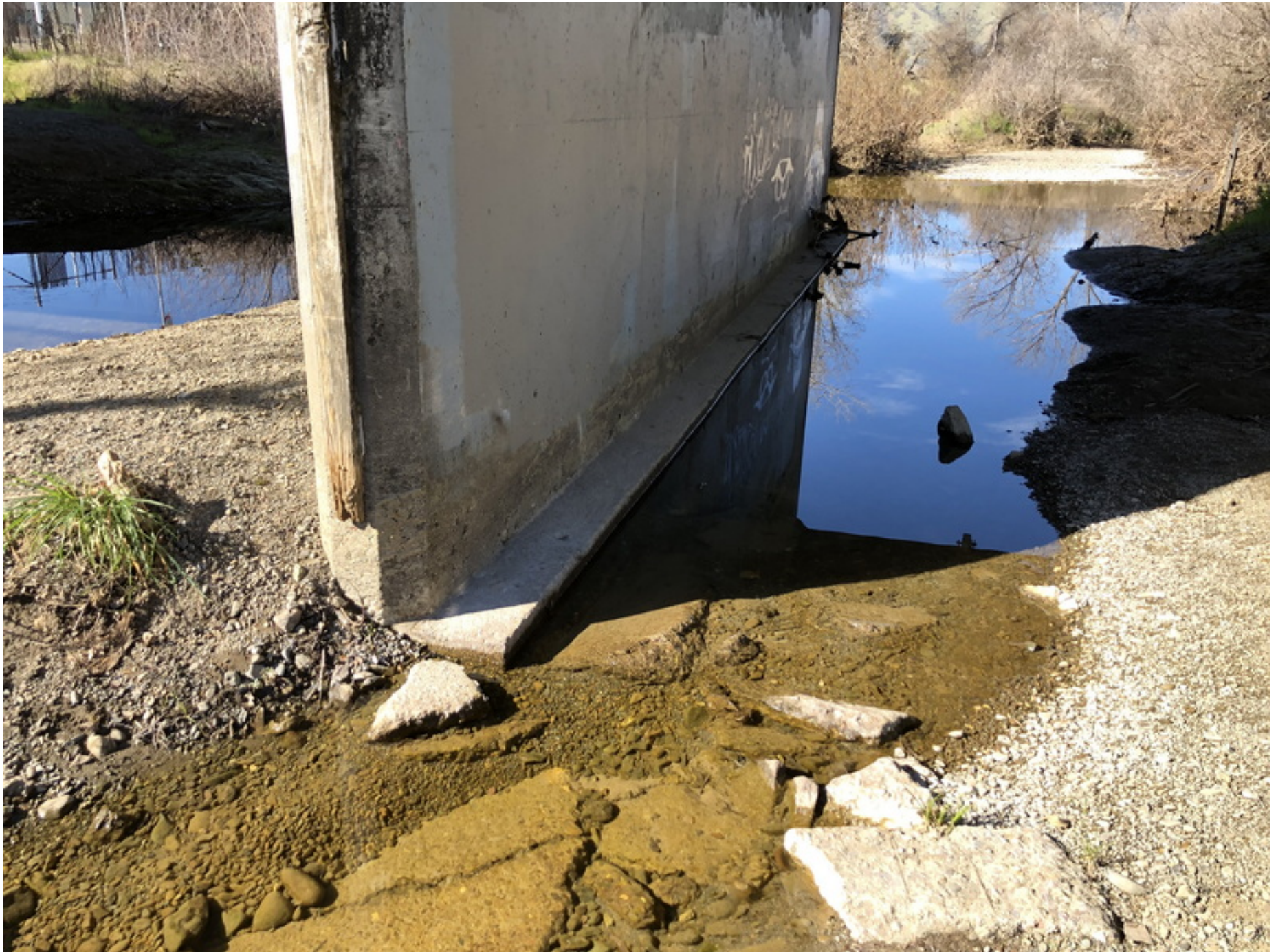
Photo #2 Showing the exposed footing from the right, downstream, end of Pier 3 (Span 3 side).
