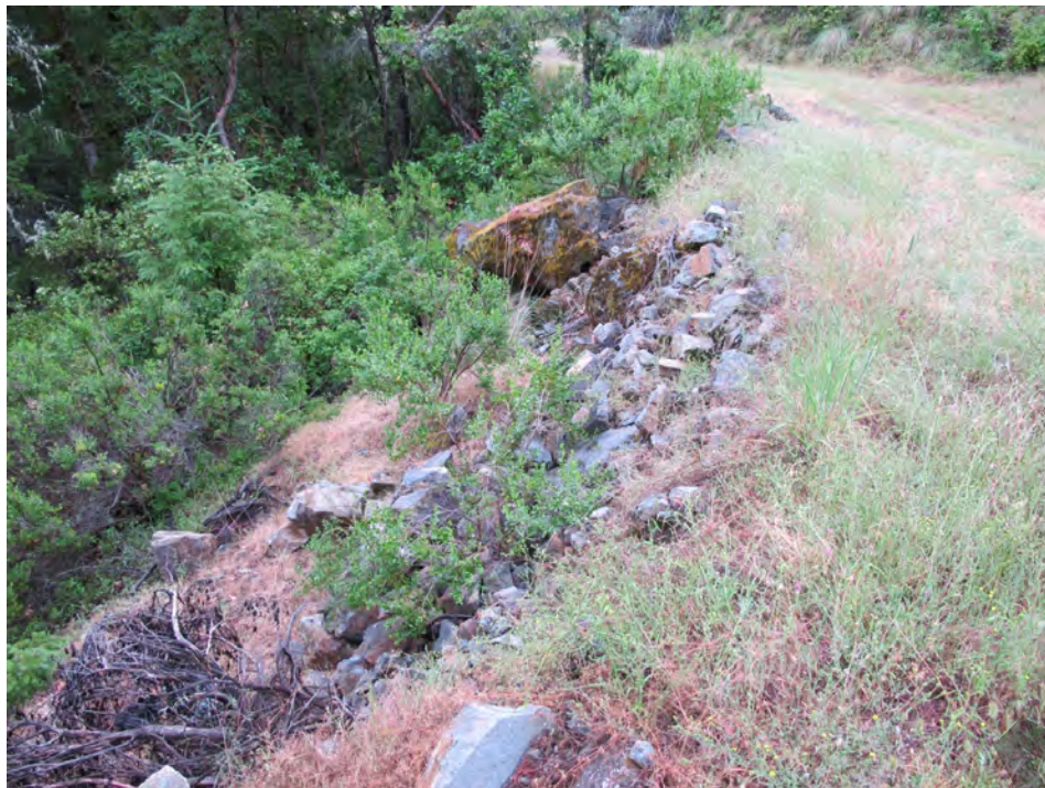
Photo Location 6: Looking east; angular crushed rock armoring 15' high fill on outboard slope, waterbar crossing road.
