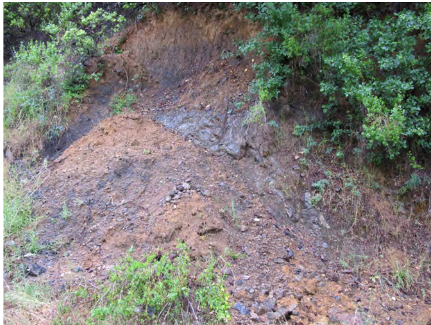
Photo Location 3b: Photo of landslide along road cut.
