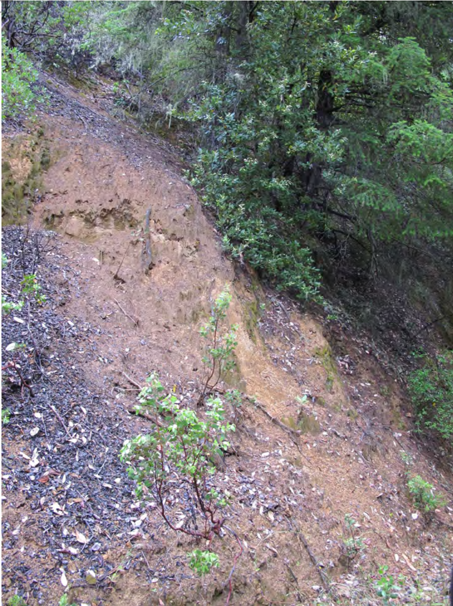
Photo Location 9: Looking north; photos of landslide(s) in and above road cut.
