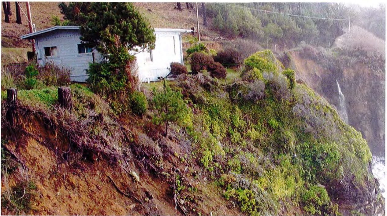
Figure 2. Landscaping and invasive vegetation along the bluff edge from the north looking south.
