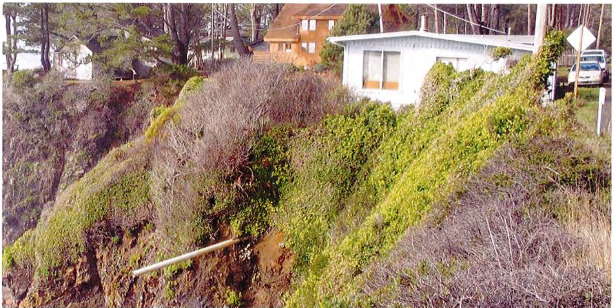
Figure 3. Landscaping and invasive vegetation along the bluff edge from the south looking north.
