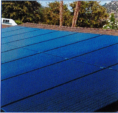
SOLAR PANEL EXAMPLE
