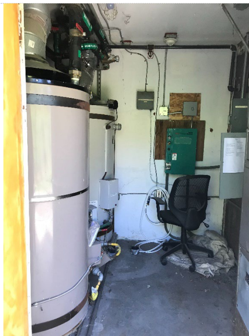
Photo #10: Electrical / Boiler Room
