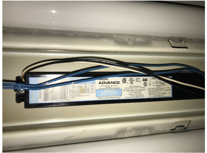
Photo #18: Ballast ICN-2P60-N No PCB's
