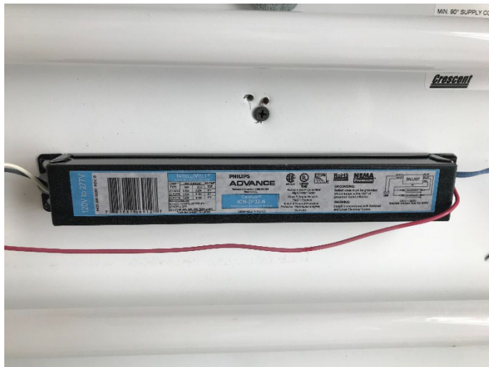
Photo #22: Ballast – ICN-2P32N No PCB's
