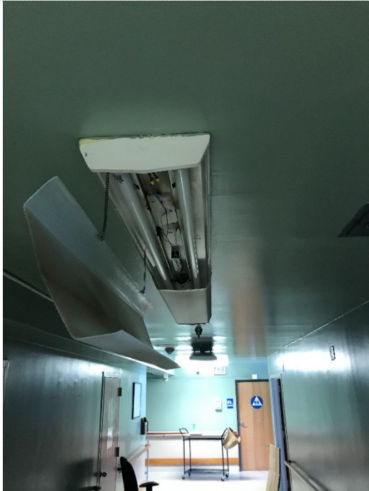
Photo #17: Ceiling light fixture
