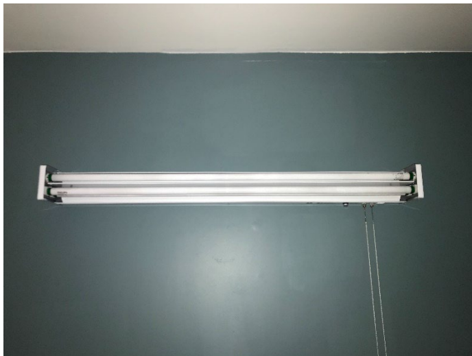
Photo #19: Wall light fixture
