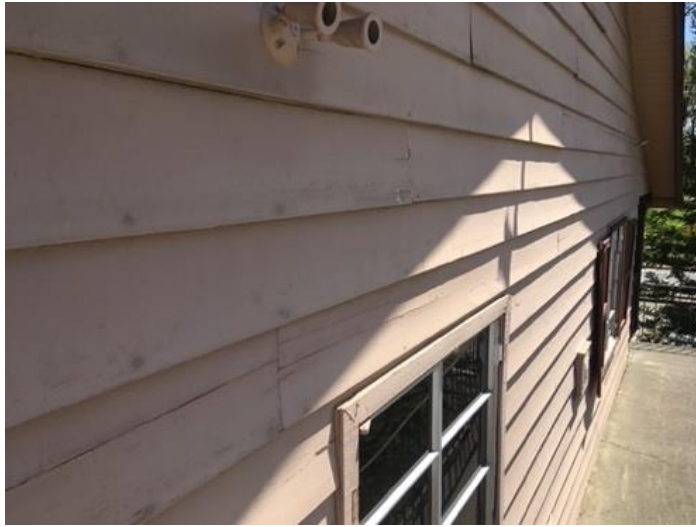
Figure 18. Detail, split siding boards at Administration Building
