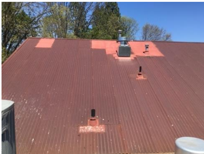
Figure 15. Corten steel roof with patched roof areas
