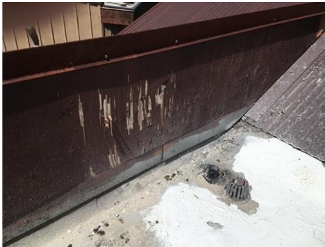
Figure 17. Detail, plywood deterioration and failed past roof patching
