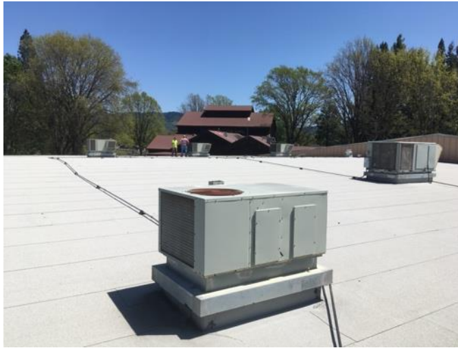
Figure 14. New roof and old rooftop HVAC units at Collections Storage Building
