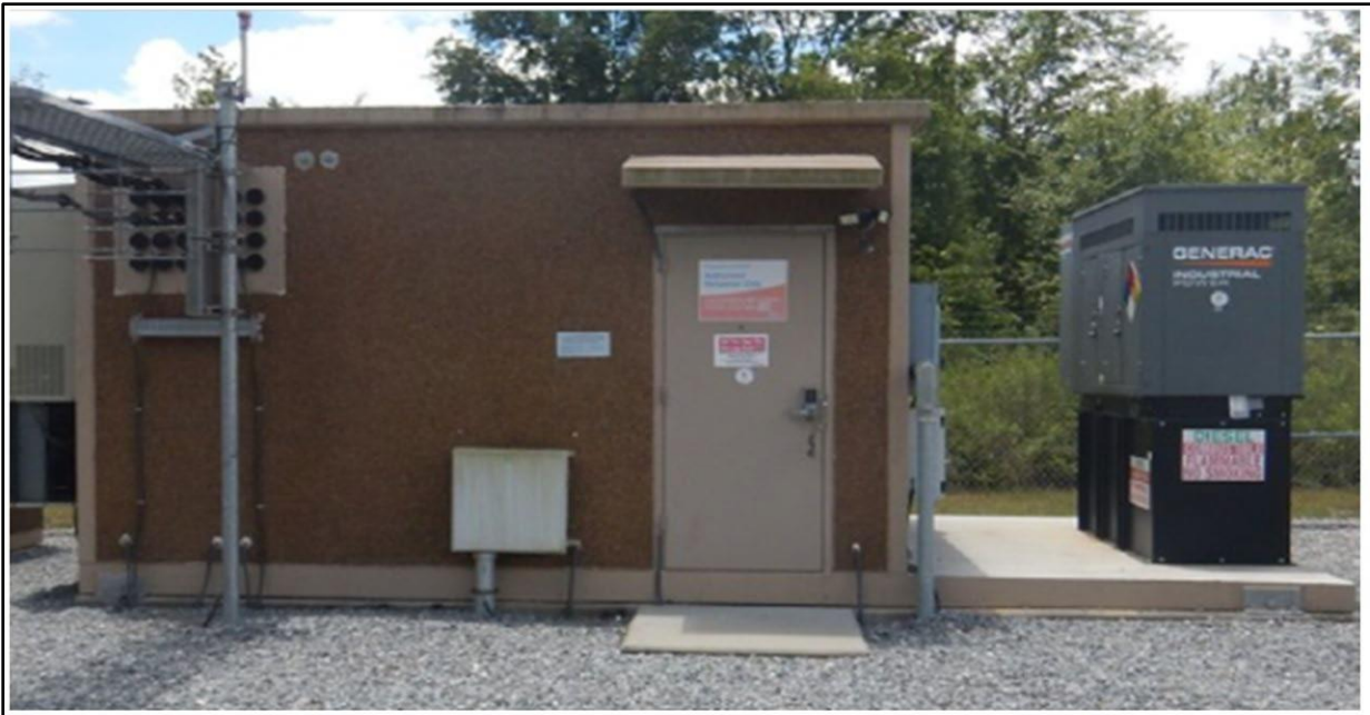
Figure 8. Network Hub with Diesel Backup Generator
