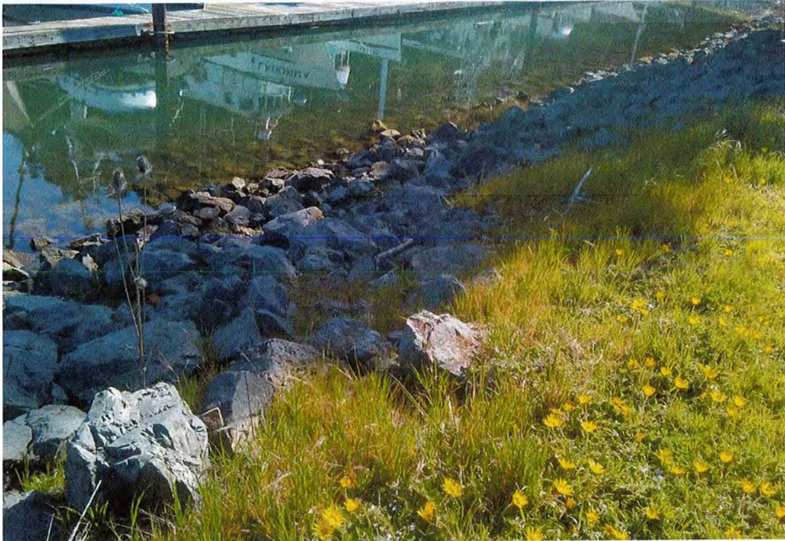
Photo 5: Looking north from top of bank to the water's edge. Note non-native species at top of bank and rip-rap on entire embankment with marina beyond. Photo taken March 31, 2022.
