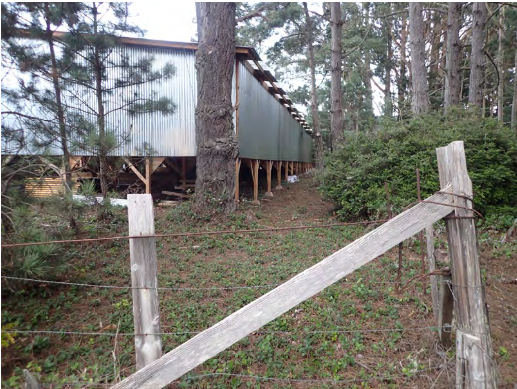
Figure 9. Southwest corner of the parcel illustrating the storage structure in relation to Bishop pine forest.
