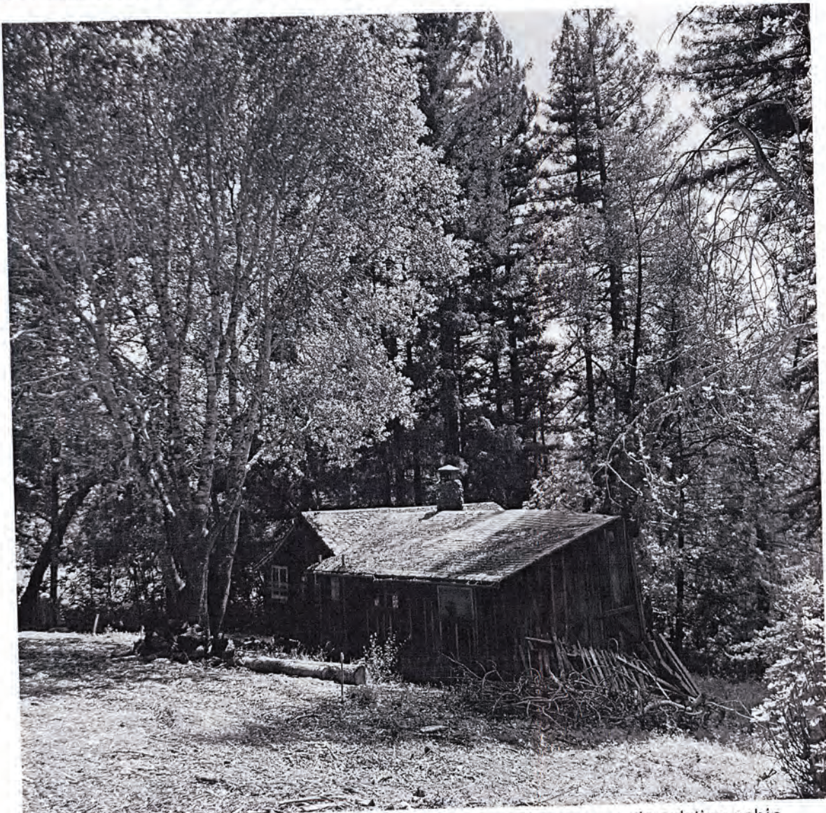
17560 Indian Creek Dr. - from front leach field easement area towards existing cabin
