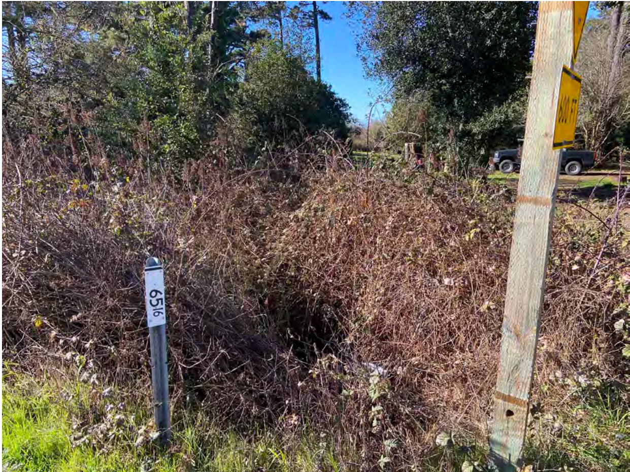
Photo Point 2. View of riparian vegetation at culvert outlet, looking west. Date of Photo: February 4, 2021.
