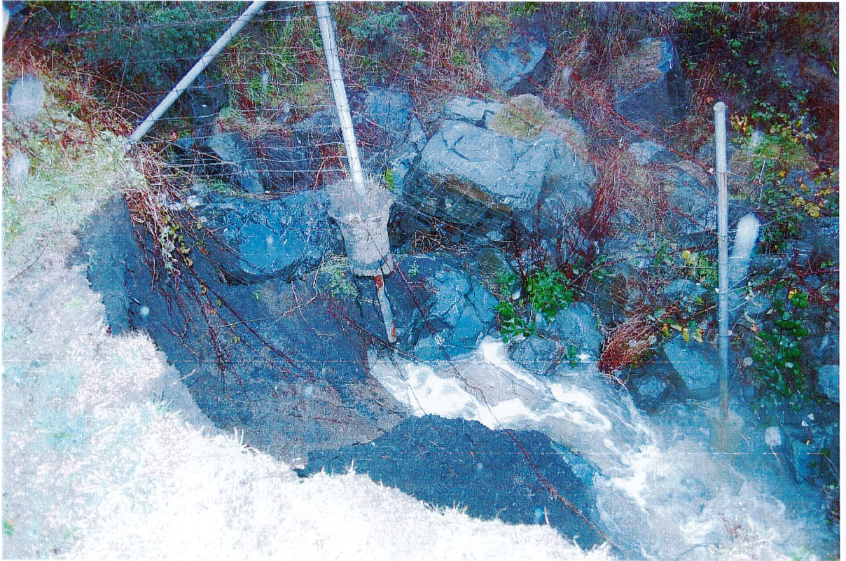
Extent of erosion by 2008 at the Cal Trans Boundary. Note that the fence shown above is, four years later, hanging in mid-air. Note the Impact on the deepening of the creek, and migration of boulders that had been added to stabilize the highway. Creek slope was eroded on our property and destabilizing the slope adjoining our driveway.
