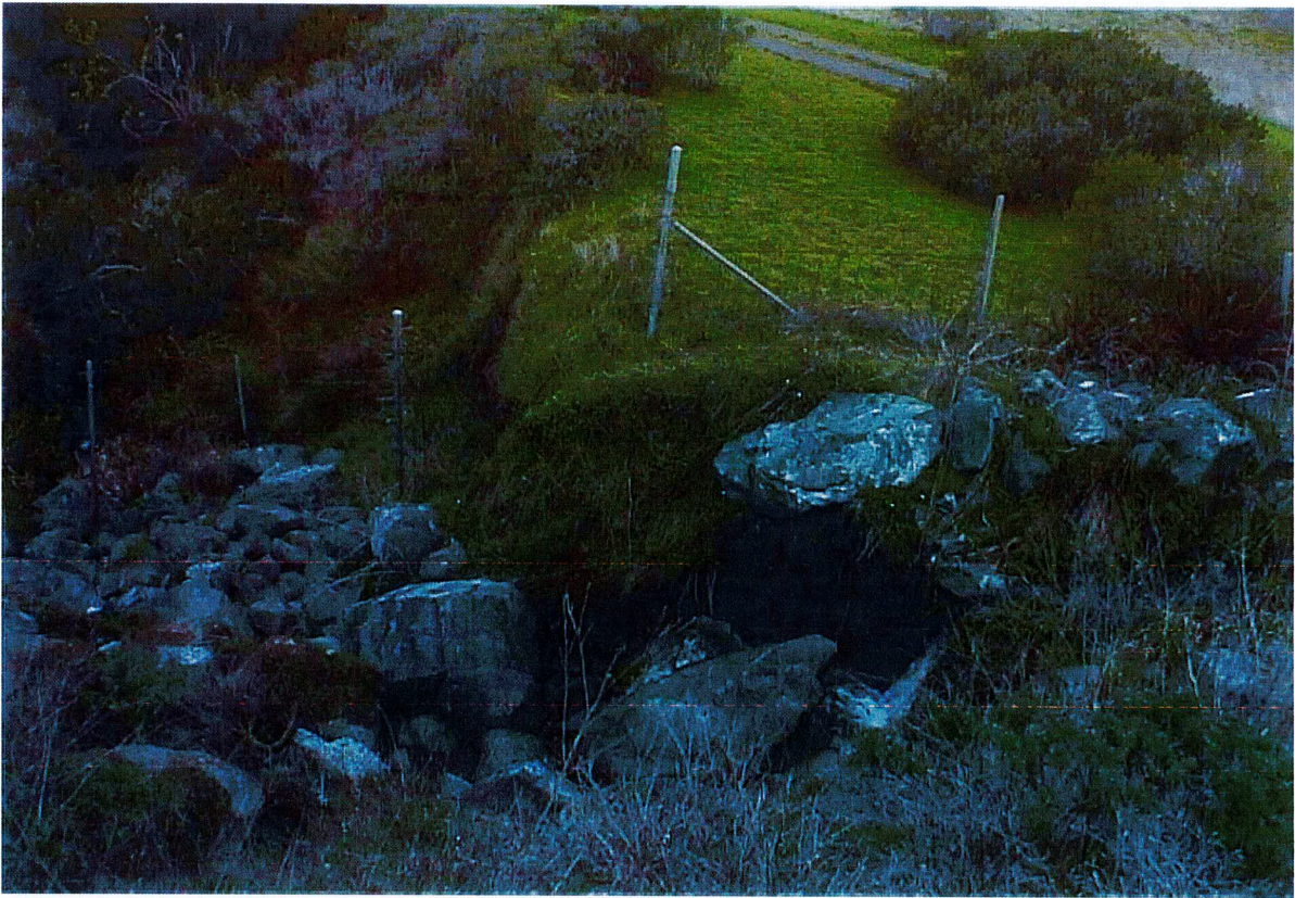
Looking from Highway One to show the extent of rock placed on the side slope of the highway. Later pictures show the rocks just sliding into the creek, actually deepening slide slopes and widening creek. Note the elevation of the CALTRANS fenceline.
