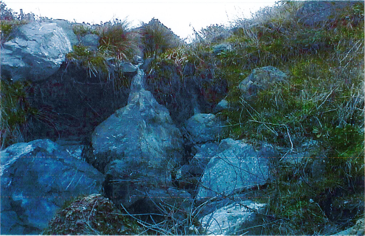
Rock revetment failing on road slope after the reconfigured drainage.
