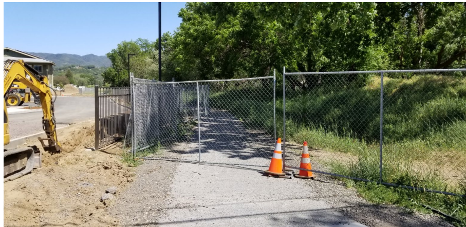
North side of Orr Street Bridge looking east along Orr Creek walking trail with fence to prevent foot traffic entry from trail to road construction. (May 2020)
