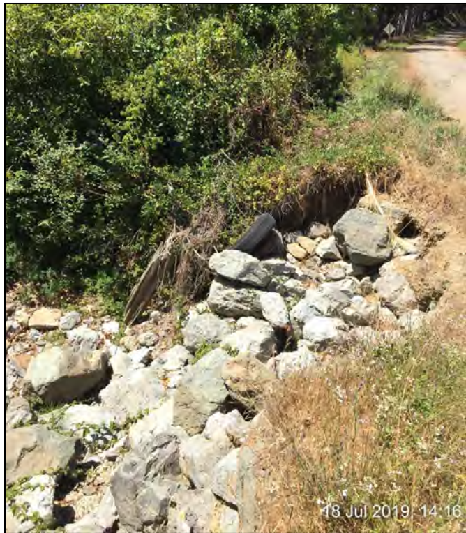
Photo 5. Looking south at Site 2, side view from the opposite end of the damages. Photograph taken July 18, 2019.
