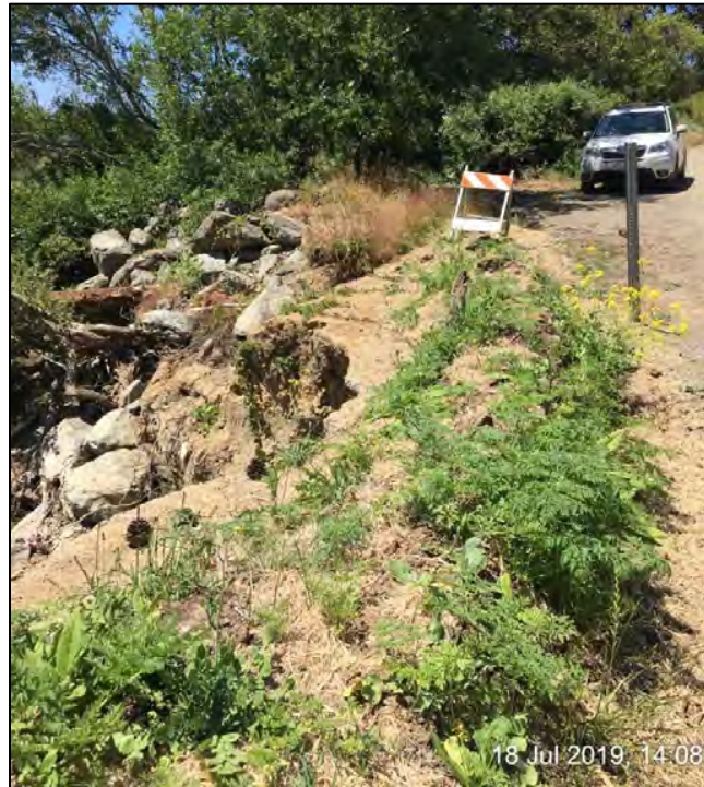
Photo 1. Facing southeast, shows the start of the damage for Site 1 where the road's shoulder and embankment was washed out. Photograph taken July 18, 2019.
