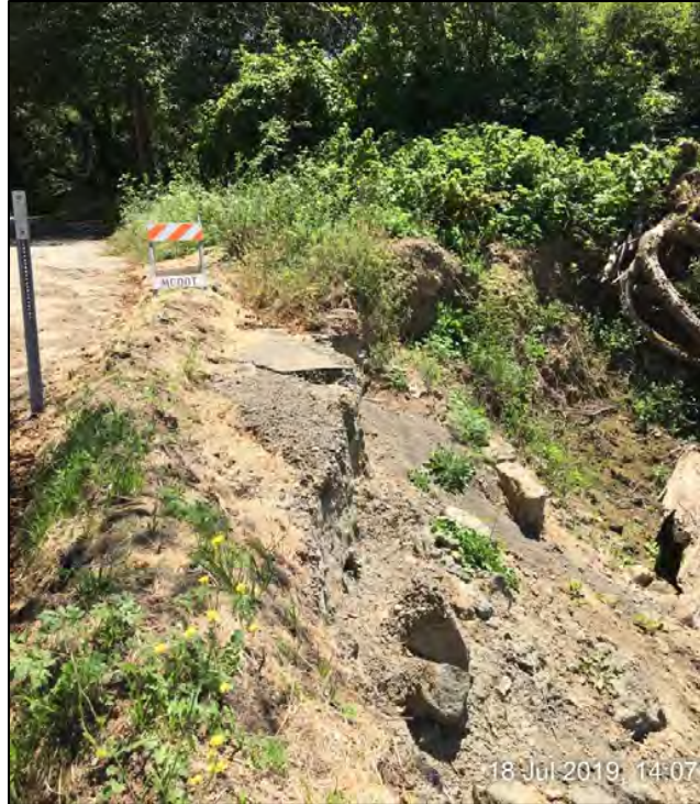
Photo 3. Looking north, the endpoint Site 1 damage. Photograph taken July 18, 2019.
