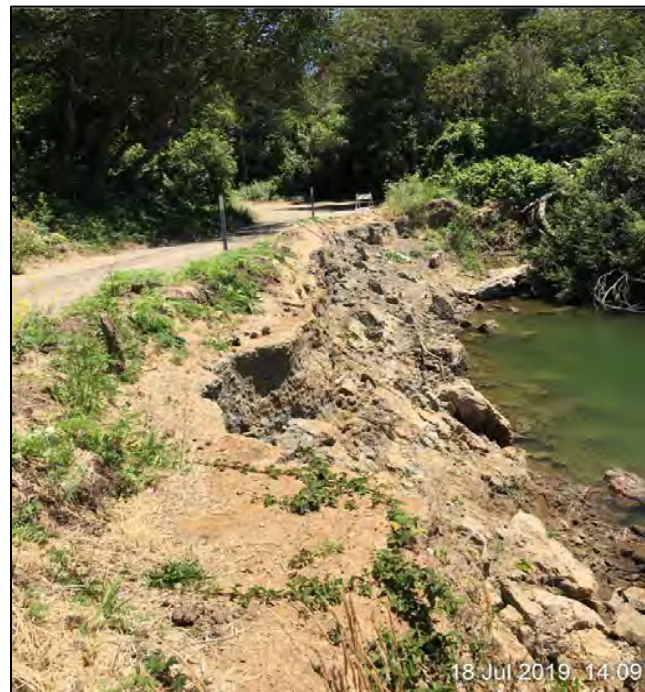
Photo 2. Looking North at Site 1, this shows the side view of the embankment shoulder where most of the washout occurred. Photograph taken July 18, 2019.
