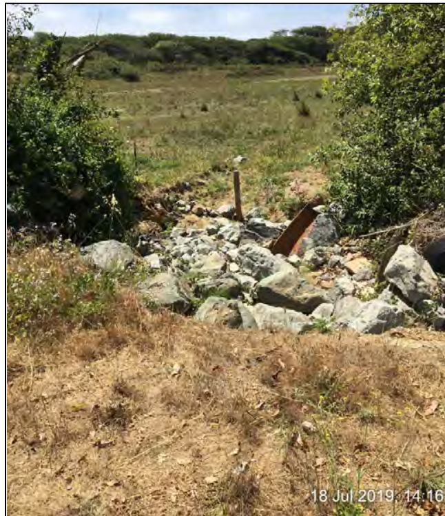
Photo 4. Facing east at Site 2, a downward view of the damage from the flooding event. Photograph taken July 18, 2019.
