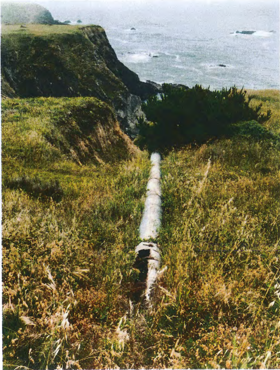
Photo 4. Culvert at PM 42.11 leading to erosional gully. Photo taken on June 13, 2019.
