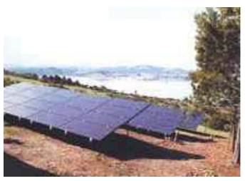
(P) SOLAR ARRAY
