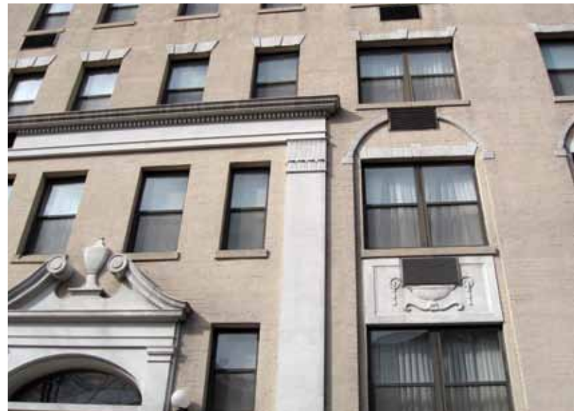
Not Recommended: [61] The cuts made in the brick and the decorative stone trim to install through-the-wall air conditioners have not only destroyed building material, but have also negatively impacted the character of this historic apartment building.
