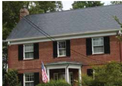
Not Recommended: [87] Historic roofing materials in good condition should be retained rather than replaced with another material perceived as more sustainable, such as, in this case, solar roofing shingles.
