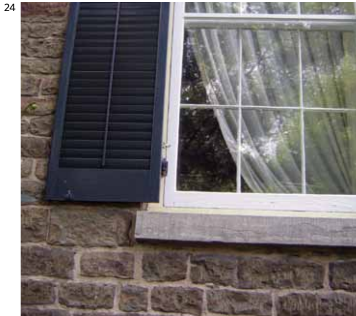
Recommended: [23-25] Historic exterior storm windows have been well maintained and continue to perform as intended.
