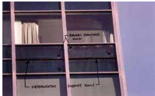
39 Recommended: [39-40] The original windows, which were deteriorated beyond repair, featured a dark tint. They were replaced with a slightly lighter-tinted glazing to improve daylighting in this mid-century modern office building.
