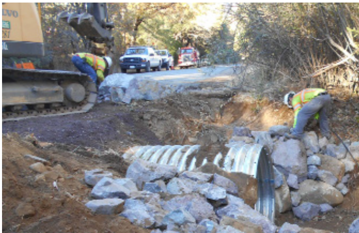
Mendocino County Department of Transportation crew working on a culvert replacement project on Eel River Road.
