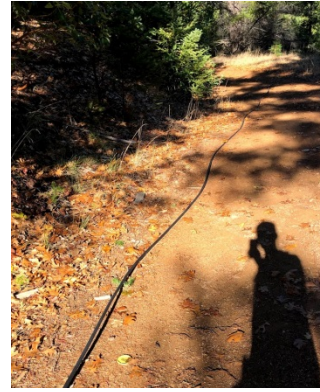
Exposed Irrigation Line
