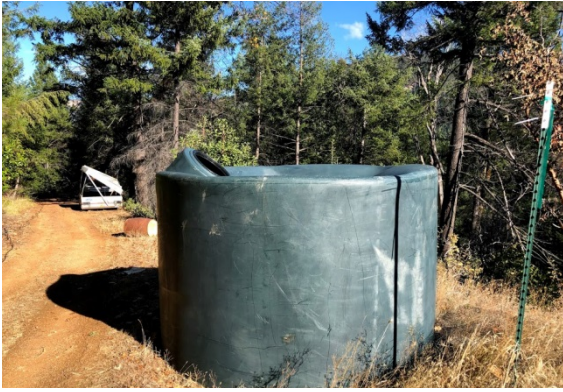
Damaged Water Tank
